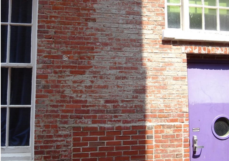
These finish remnants found on the west facade record the stone color that was once found on the exterior of the Free Street Baptist Church.
